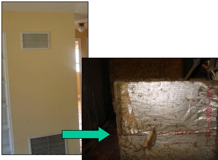
LR side of AHU closet
