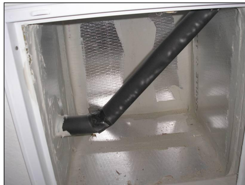
Central return plenum constructed with duct board & sealed with mastic at edges, seams, & joints.
